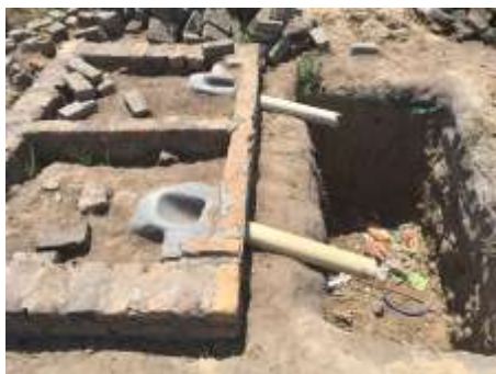
Figure 7: Two Cabin toilet under construction in Stoneridge (Picture by Mark Harper, Welthungerhilfe)
