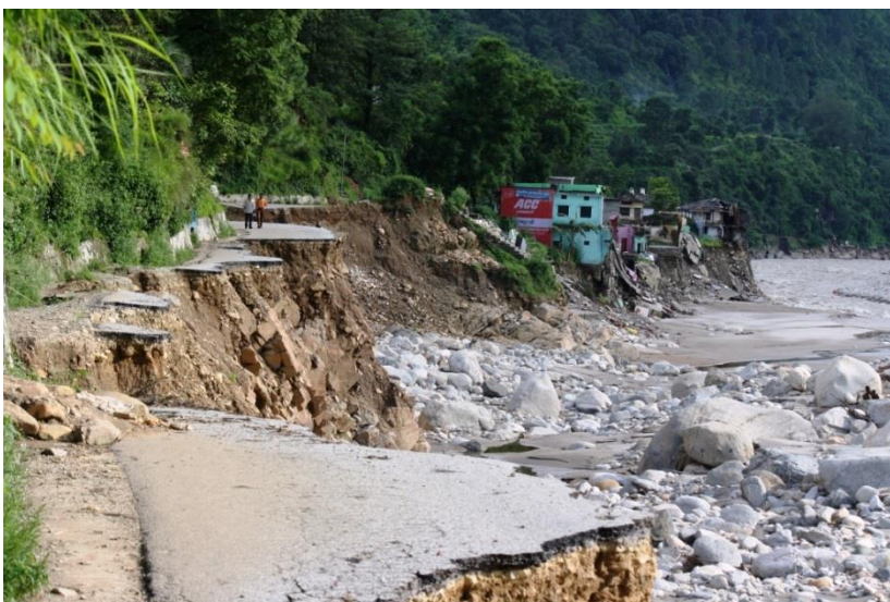
Figure 2: Severe damage to the Roads has adversely affected the Market Systems
